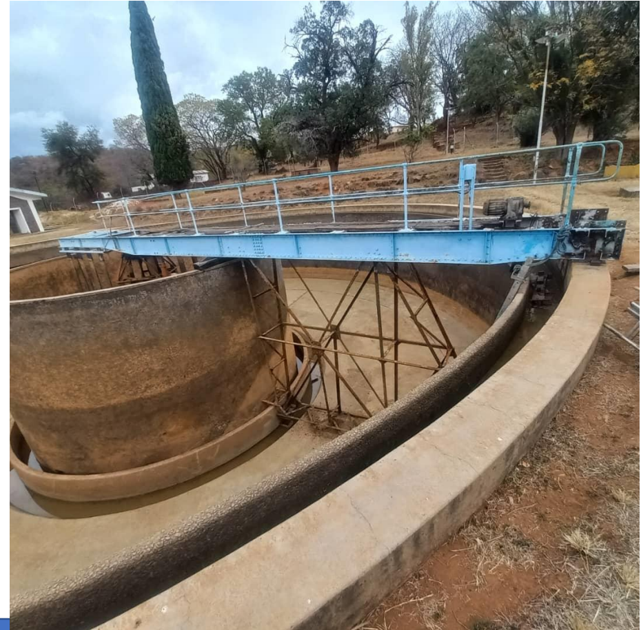
NCEMA WATER WORKS CLARRIFIER NO. 2
